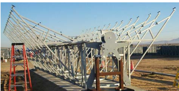
Figure 3: Space frame of a EuroTrough module with measurement targets on the mirror support points
