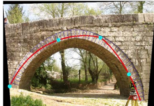
Figure 7. Graphic results of the structural analysis. Representation of the thrust line as well as the four-hinges mechanism.
