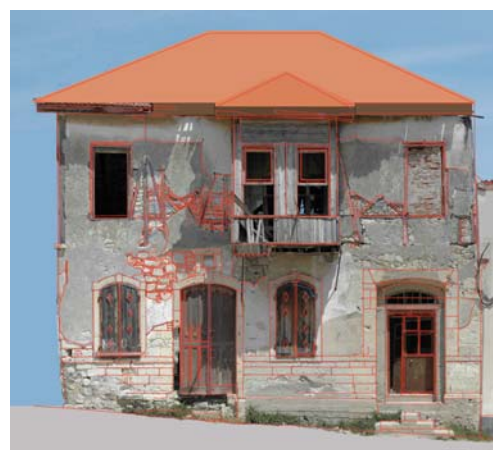
Figure 5. The orthoimage of the southern façade, overlapped with the 2D scaled drawing
